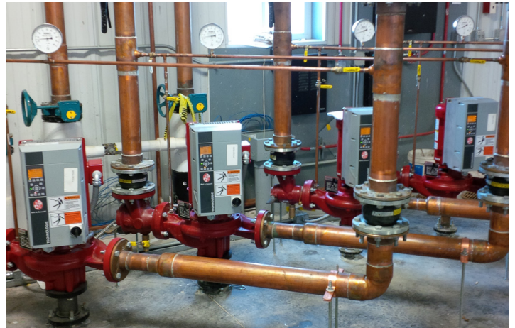
Series e-80 pumps installed with Technologic IPC variable frequency drive and Technologic PPS controller
